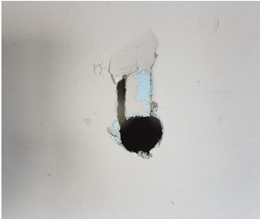
Plate 7. B1- High suitability to support roosting bats, internal view. Damage to internal walls; small hole in wall.
