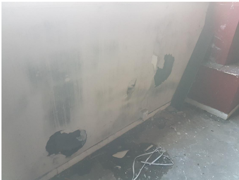
Plate 8. B1- High suitability to support roosting bats, internal view. Damage to internal walls; multiple holes in wall below window.
