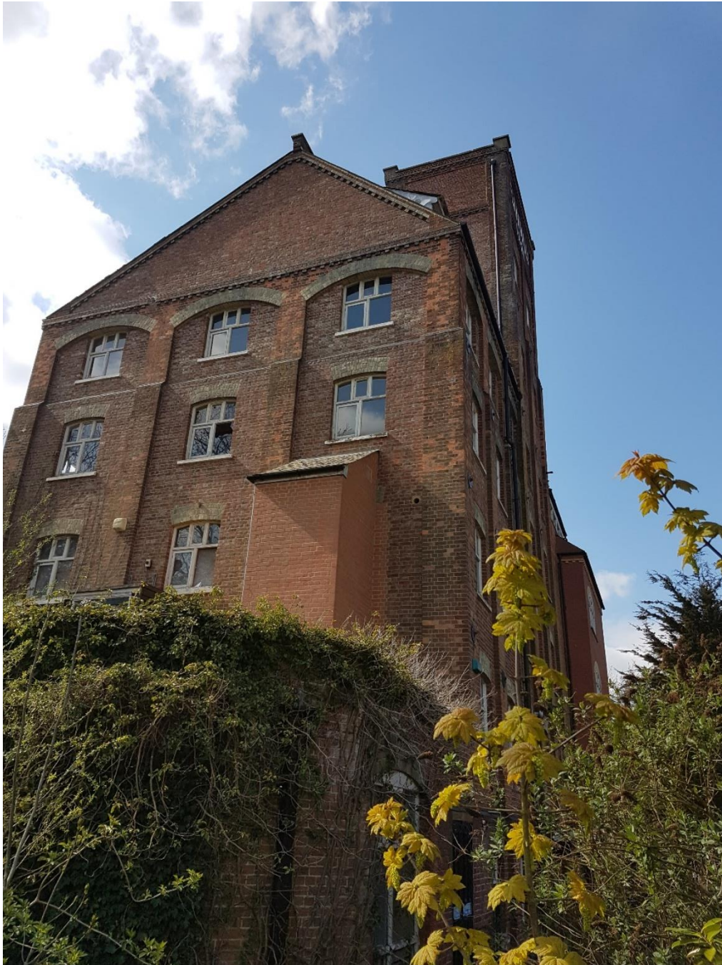
Plate 14. B1- High suitability to support roosting bats, external view. Broken windows along the northern face of the building. Common ivy covers the northern face of building. Not pictured; common ivy covering the eastern face of the building.
