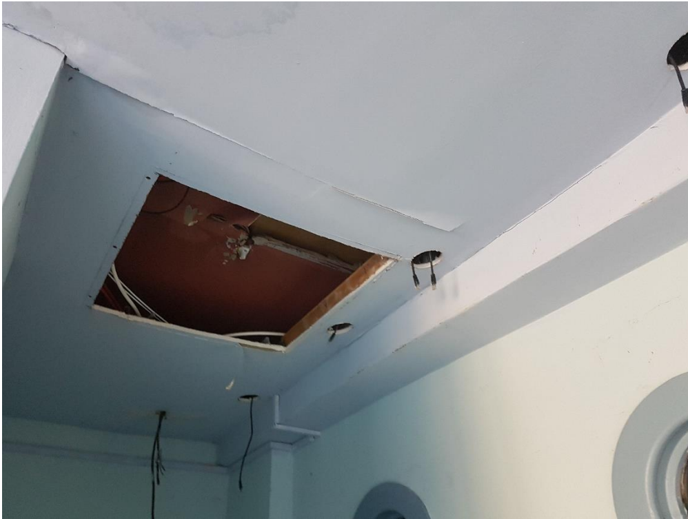
Plate 9. B1- High suitability to support roosting bats, internal view. Potential access into roof, above plasterboards through hole in the ceiling from unused lights and roof access.
