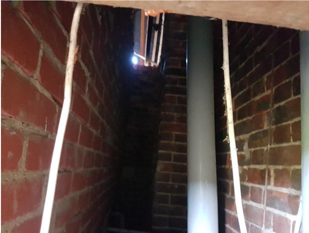
Plate 3. B1- High suitability to support roosting bats, internal view. Additional cavities present in and behind walls, blocked from sunlight.
