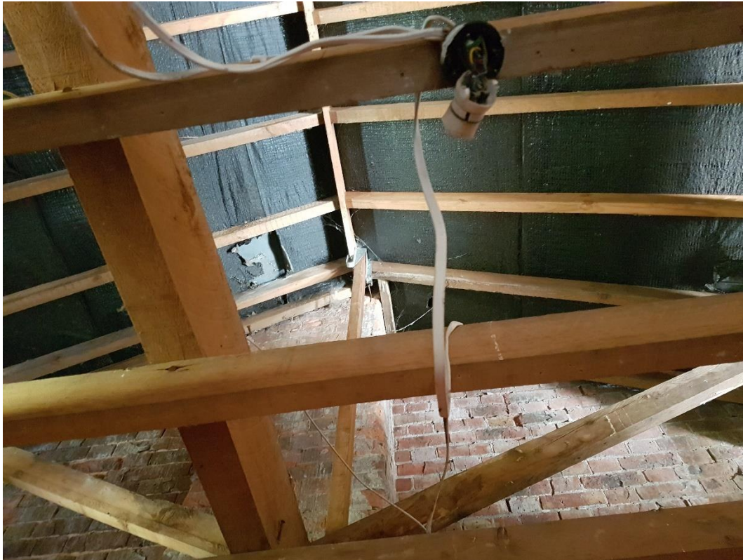
Plate 5. B1- High suitability to support roosting bats, internal view. Holes in bitumen felt lining.
