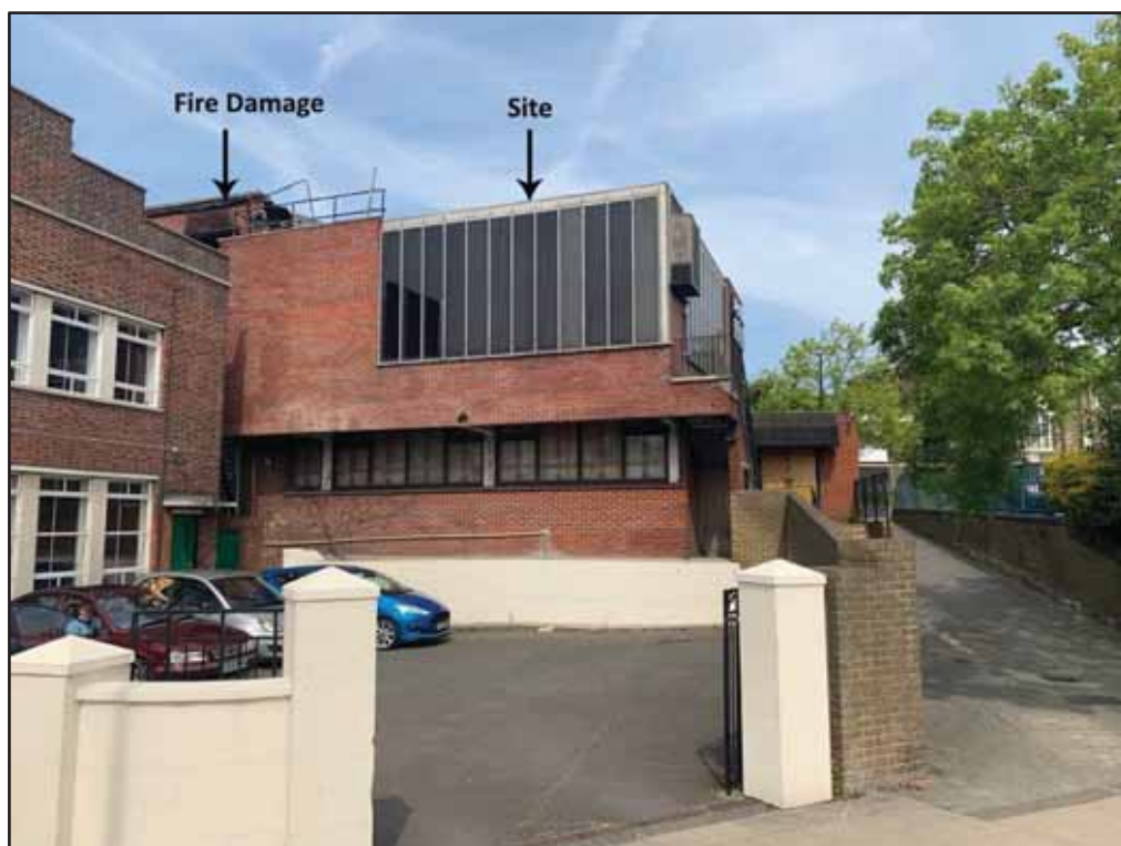
Image 22: View northeast from Snargate Street showing fire damage to roof
